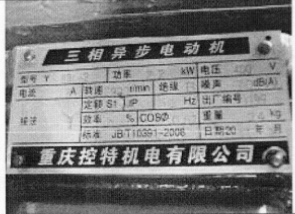
Photo 4. Three phase motor
